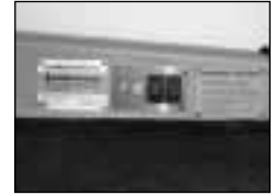
Photo #2 Control Panel
